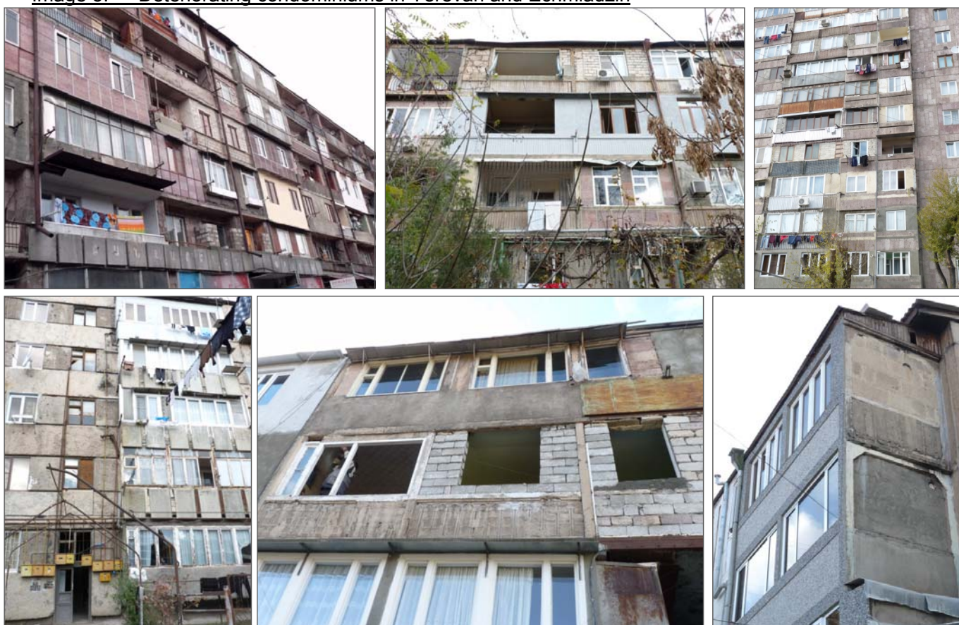
Image 5: Deteriorating condominiums in Yerevan and Echmiadzin
