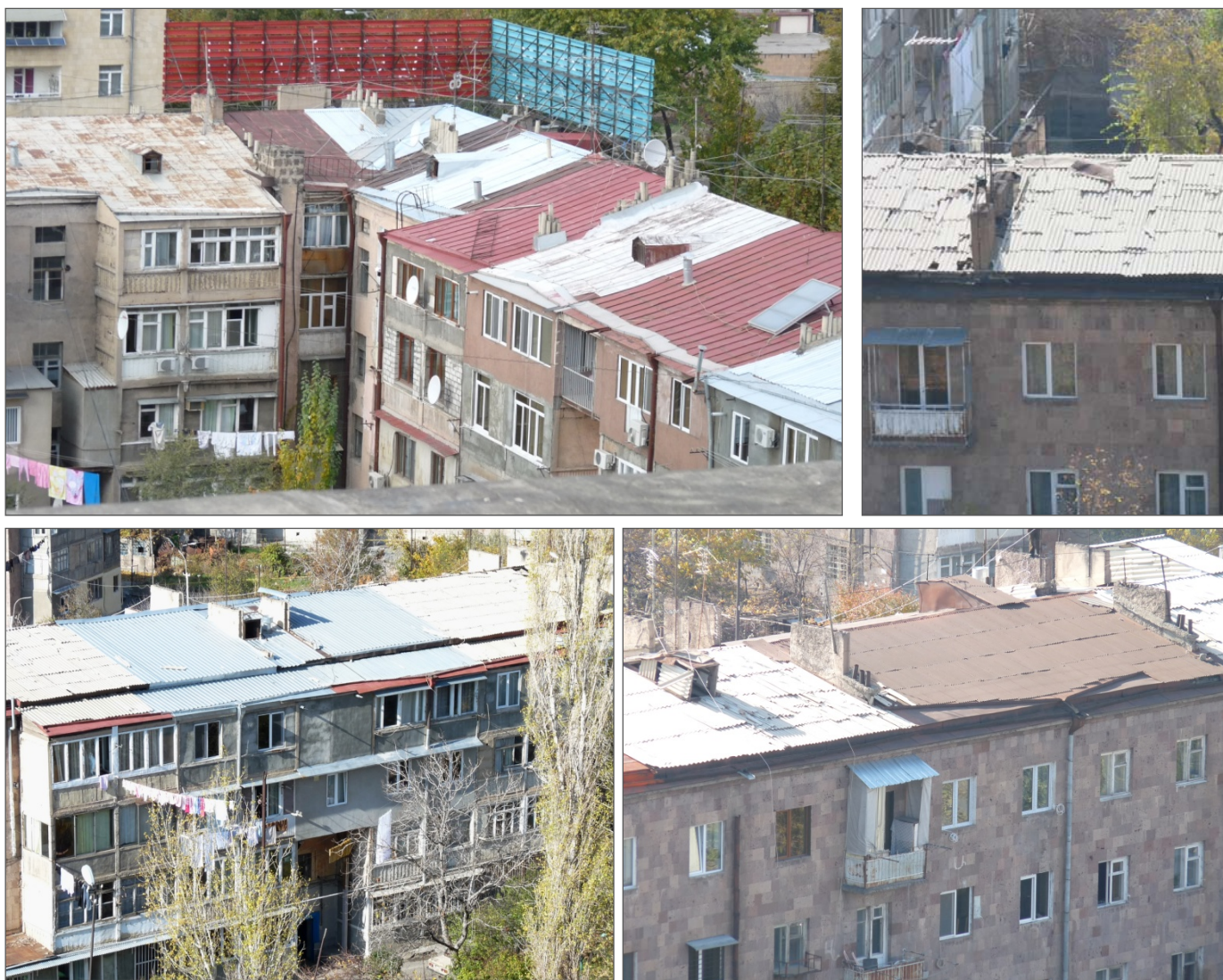
Image 7: Condominium in Yerevan – prior complaint: roofs
