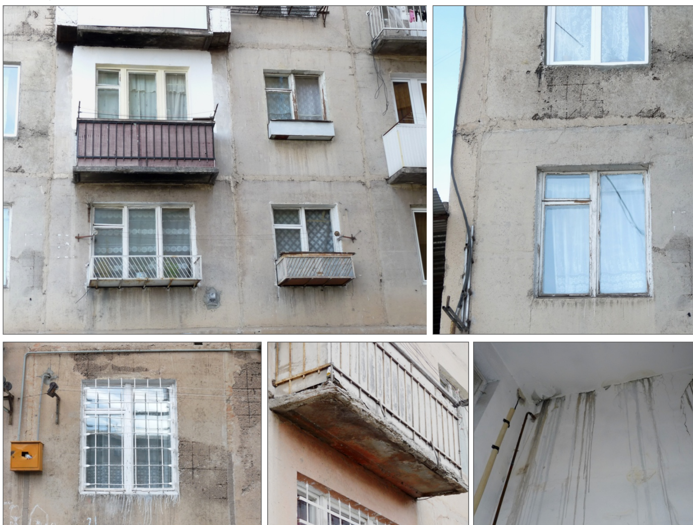
Image 6: Condominium in Yerevan – poor condition of panel block construction
